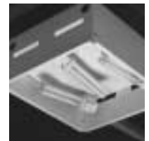
After mounting frame is installed, entire unit can be wired and lamped, then lifted into plenum.
